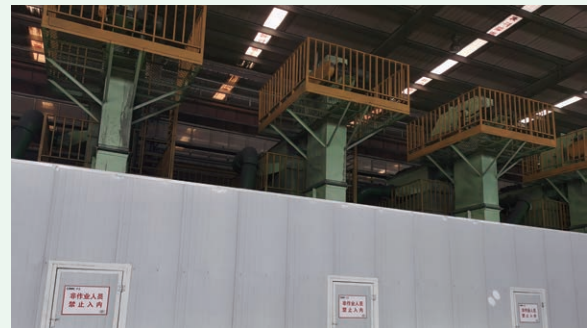
厚板线打砂机隔音墙
